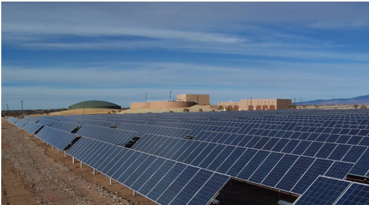
Photo 1 Buckman Direct Diversion Solar Array
